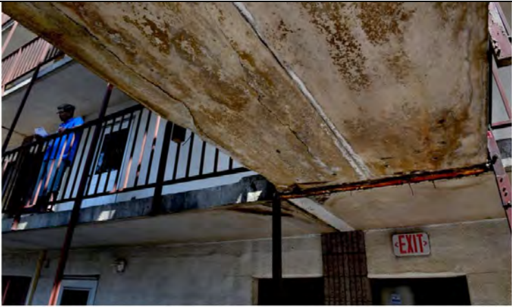
The crumbling walkway on the second floor at Hermitage Woods. The elevator in the aging five-story complex hasn't worked for at least six months. Parts of the wraparound balcony are cordoned off because of structural weakness. (Michael S. Williamson/The Washington Post)
