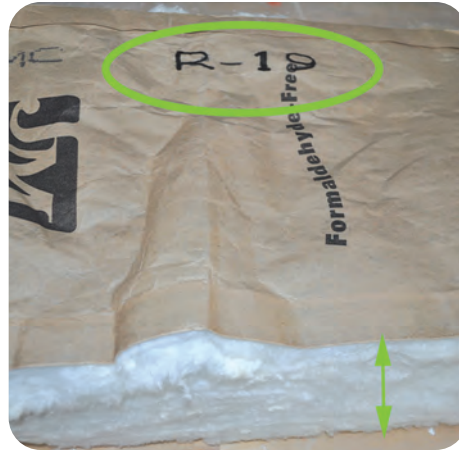
2. Insulation R-value matches work order
