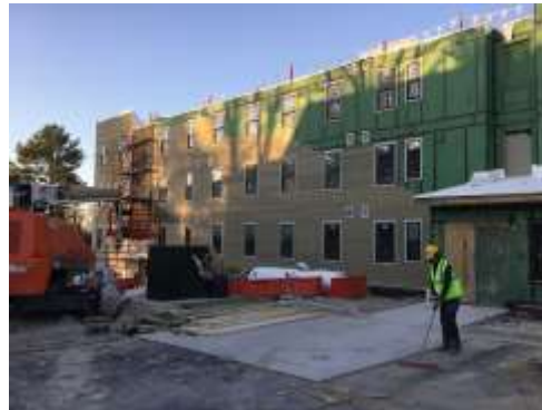
Figure 2 In progress new construction for Restoration Gardens 2, FY2016 RFA award of $250,000 for demolition
